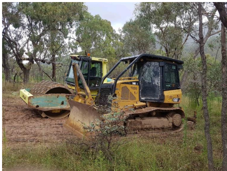
Figure 5: Unprecedented resources were put into roadworks on NVFT late in the 2021/22 goanna season, with seven major plant units operating in two areas of the NVFT at once
