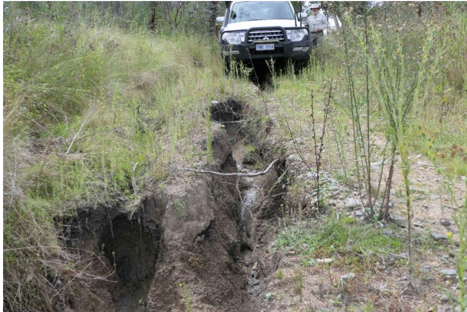
Figure 4: Tarweed in the middle section of NVFT with deep rills threatening to cut the road.
